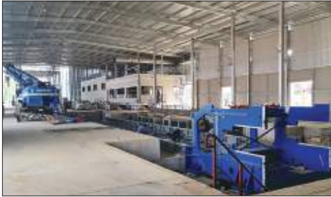
The CPS+ continuous press, the centerpiece of the new DIEFFENBACHER MDF plant for Wisewoods Co. Ltd. in Khao Yoi, Phetchaburi, Thailand, is currently under construction.
